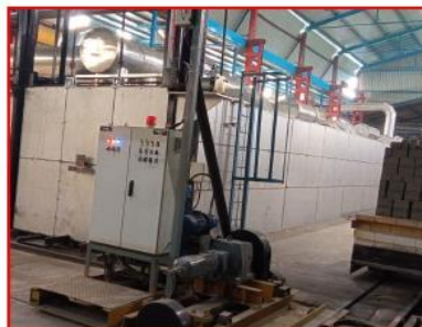
HIGH ALUMINA TUNNEL DRYER
