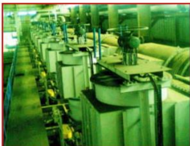
GRAPHITE ELECTRODE REBAKE TUNNEL KILN
