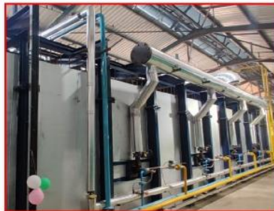
HIGH TEMPERATURE TUNNEL KILN
